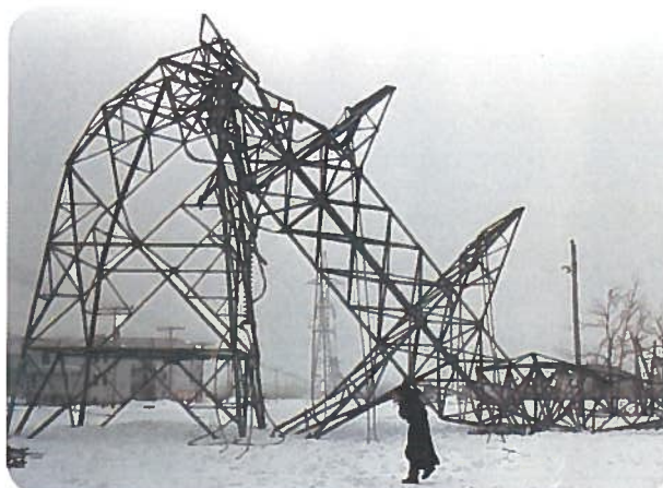
Figure 9 Transmission towers toppled from the weight of the ice. Previously, the worst ice storm on record was in 1961. In that case, only 60 mm of ice accumulated and lasted only a day or two.
