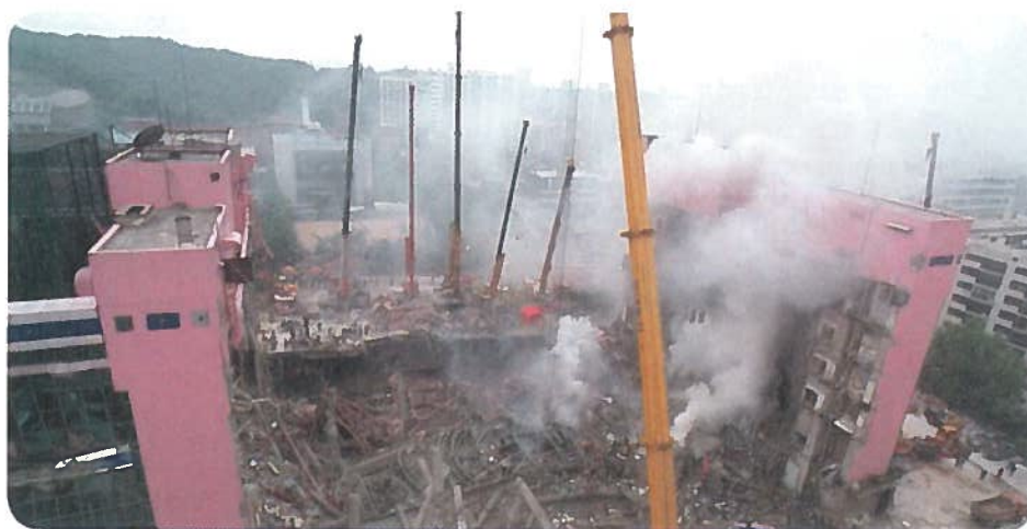
Figure 8 The remains of the Sampoong Department Store after its collapse
