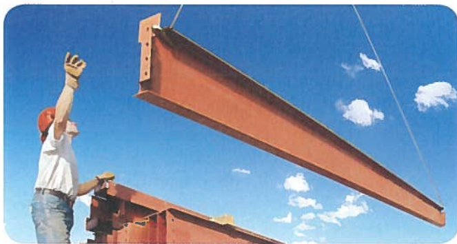
Figure 2 A steel I-beam is used to provide structural strength.
