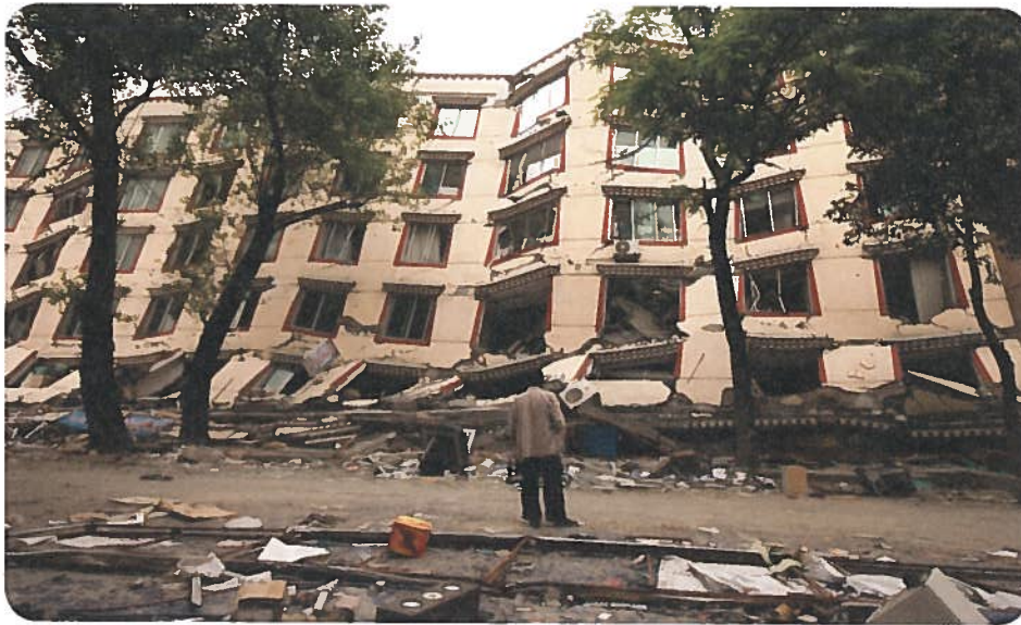
Figure 1 This building was destroyed by the earthquakes in Sichuan Province, China, in 2008.
