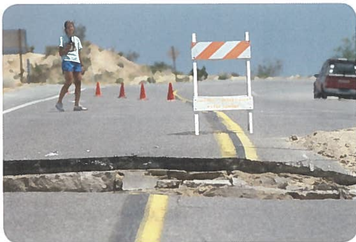
Figure 1 This road failed because of shear forces. An earthquake caused the two sides of the road to slide in opposite directions.
