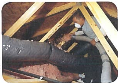
Figure 2 Insulation is put into the walls and roof of a house to prevent the transfer of energy.
