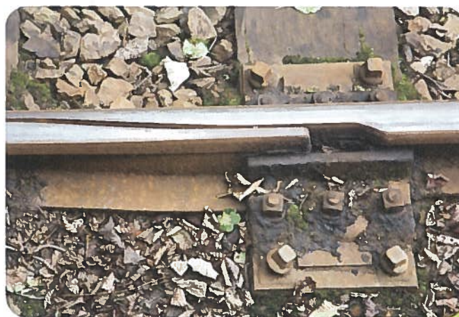
Figure 2 A breather switch. The sharp angle at which rails are cut ensures a relatively smooth and quiet ride for passengers.
